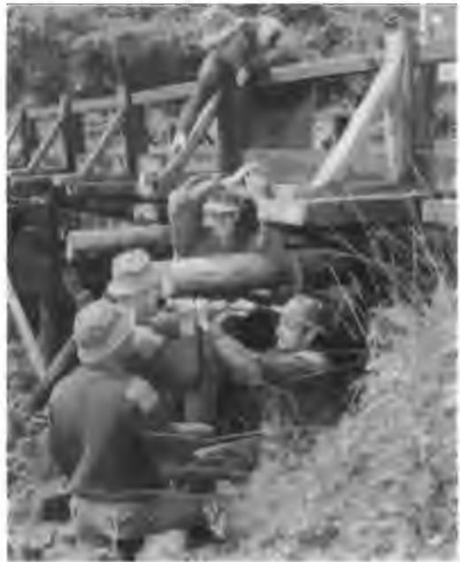
The Assault Pioneers repairing a bridge whilst exercising at Gathuru in Kenya.
